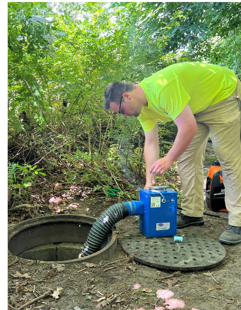
Massachusetts Maritime Academy coop student conducting a smoke test to help map a stormwater network and detect potential illicit connections. Photo by Kathleen Kutschenreuter for the U.S. EPA
