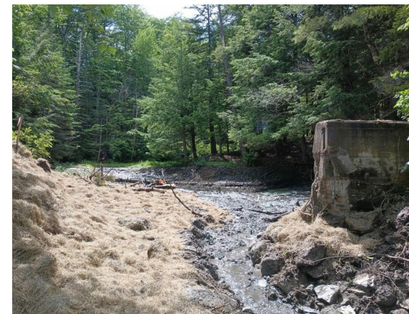
Frost Gully Dam on Frost Gully Brook in Freeport, Maine, following breaching and partial removal.
