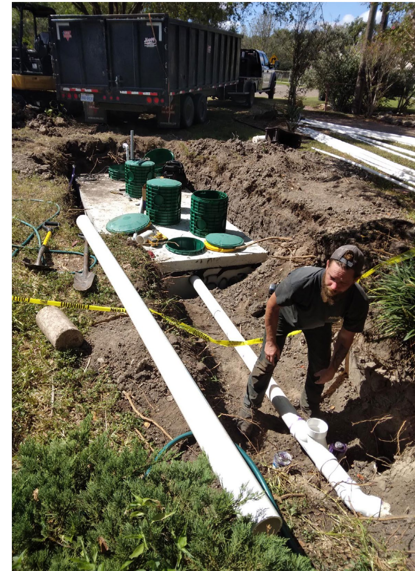
A contractor installing on-site sewage facilities replacements implemented by the Coastal Bend Bays & Estuaries Program's OSSF Assistance Program.
