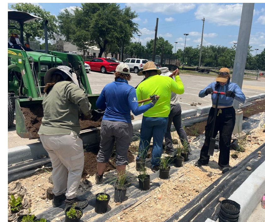
Houston Parks and Recreation Department staff and volunteers planting native plants in a newly created bioswale at Townwood Park in southwest Houston, Texas. This bioswale collects and cleans water from the parking lot before it flows into Sims Bayou. Photo by the Galveston Bay Estuary Program
